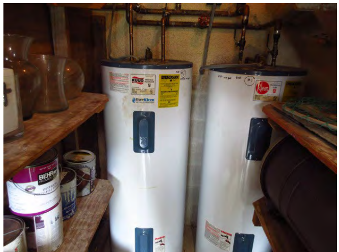
VIEW OF WATER HEATERS
