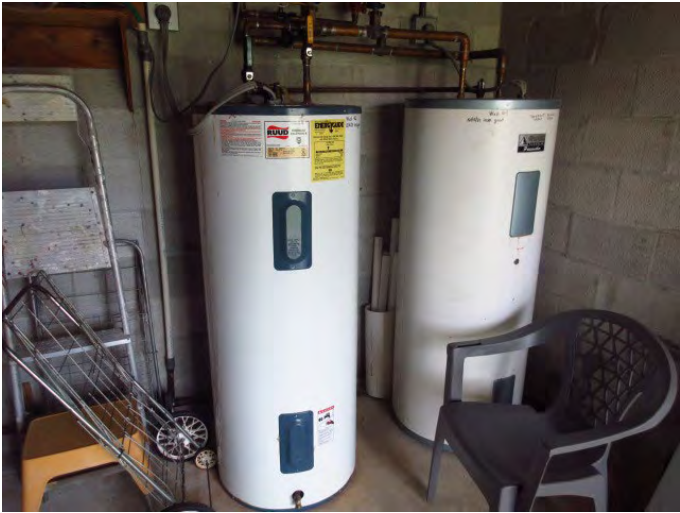
VIEW OF WATER HEATERS
