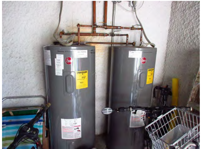
GENERAL VIEW OF DOMESTIC WATER HEATERS
