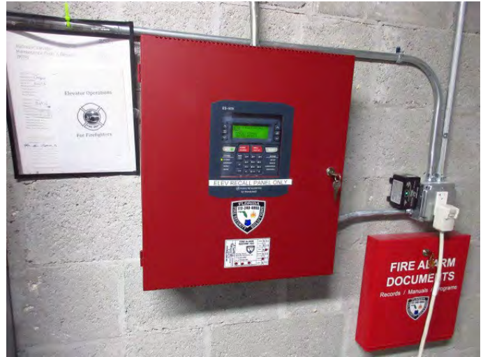
VIEW OF CENTRAL ALARM PANEL
