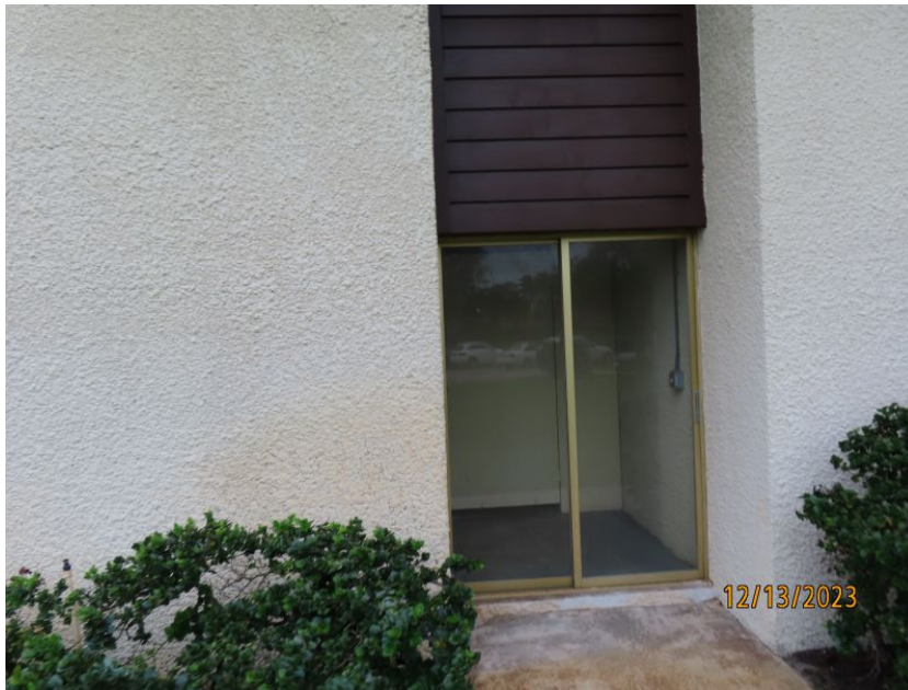
Unprotected Glazed Entry Door
