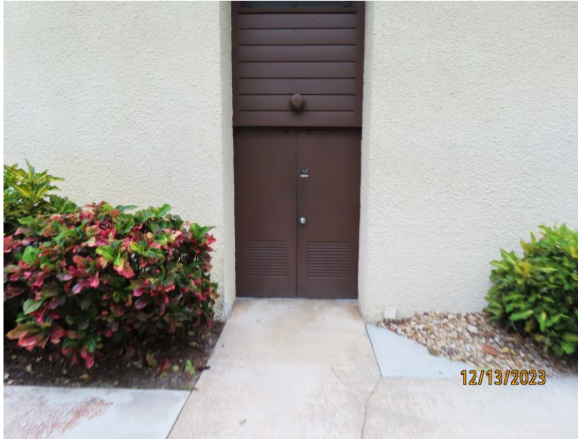
Unprotected Solid Entry Door
