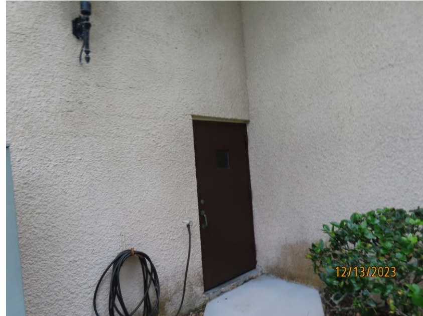
Unprotected Solid Entry Door
