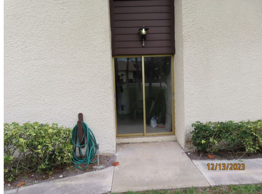
Unprotected Glazed Entry Door
