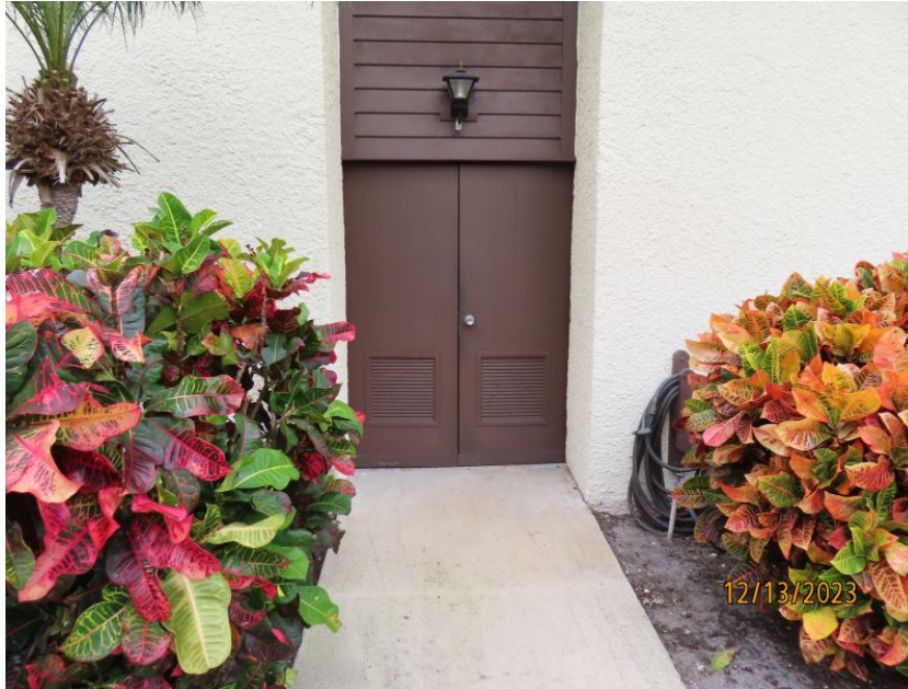
Unprotected Solid Entry Door
