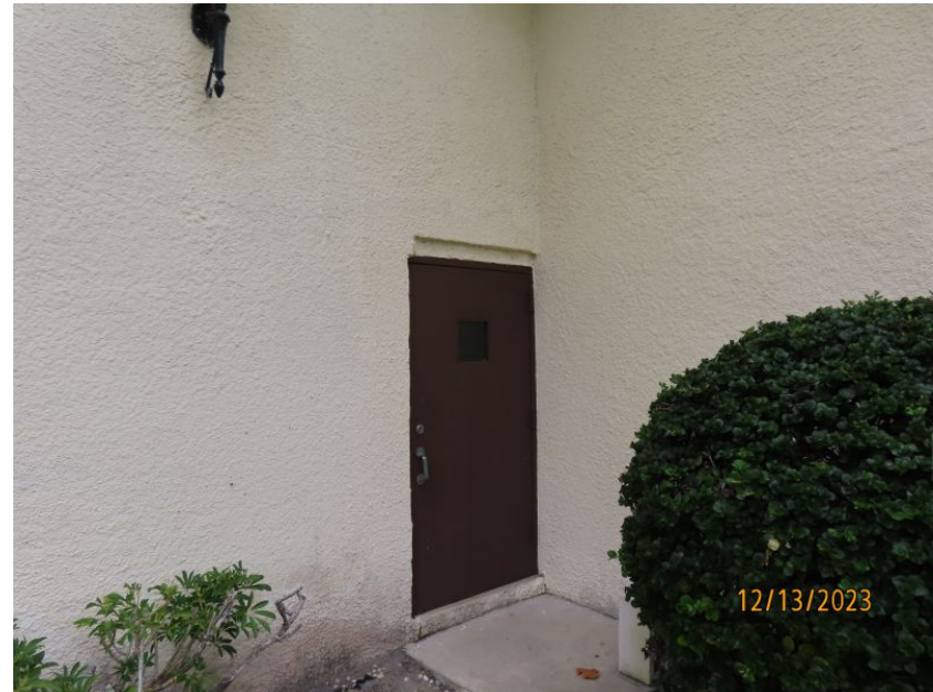
Unprotected Glazed Entry Door
