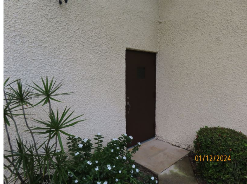
Unprotected Glazed Entry Door
