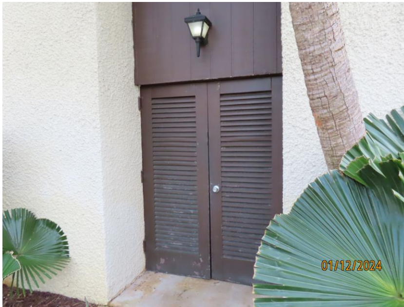
Unprotected Solid Entry Door
