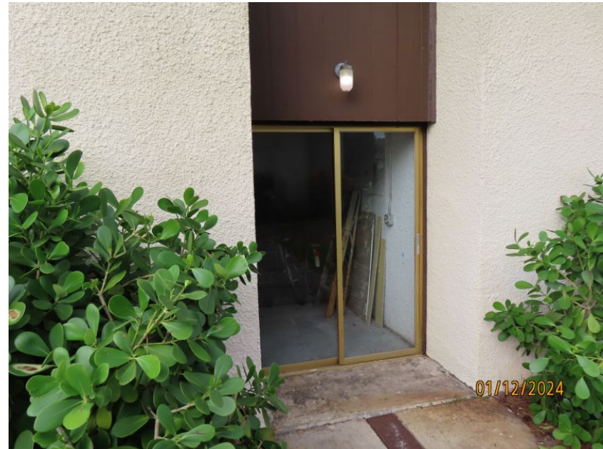
Unprotected Glazed Entry Door
