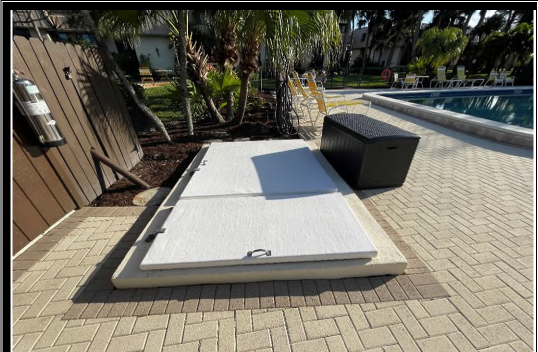
VIEW OF TYPICAL POOL EQUIPMENT
